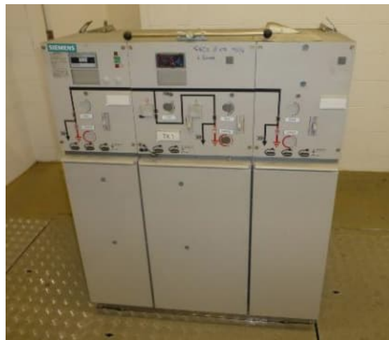
RLR in an indoor substation
