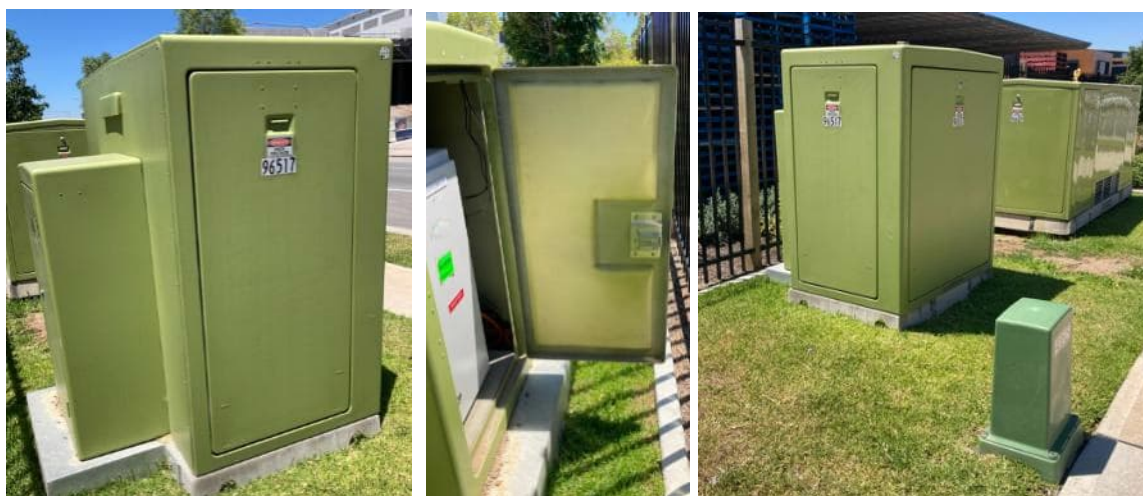
Photos of switching station cubicle with RTU cubicle
